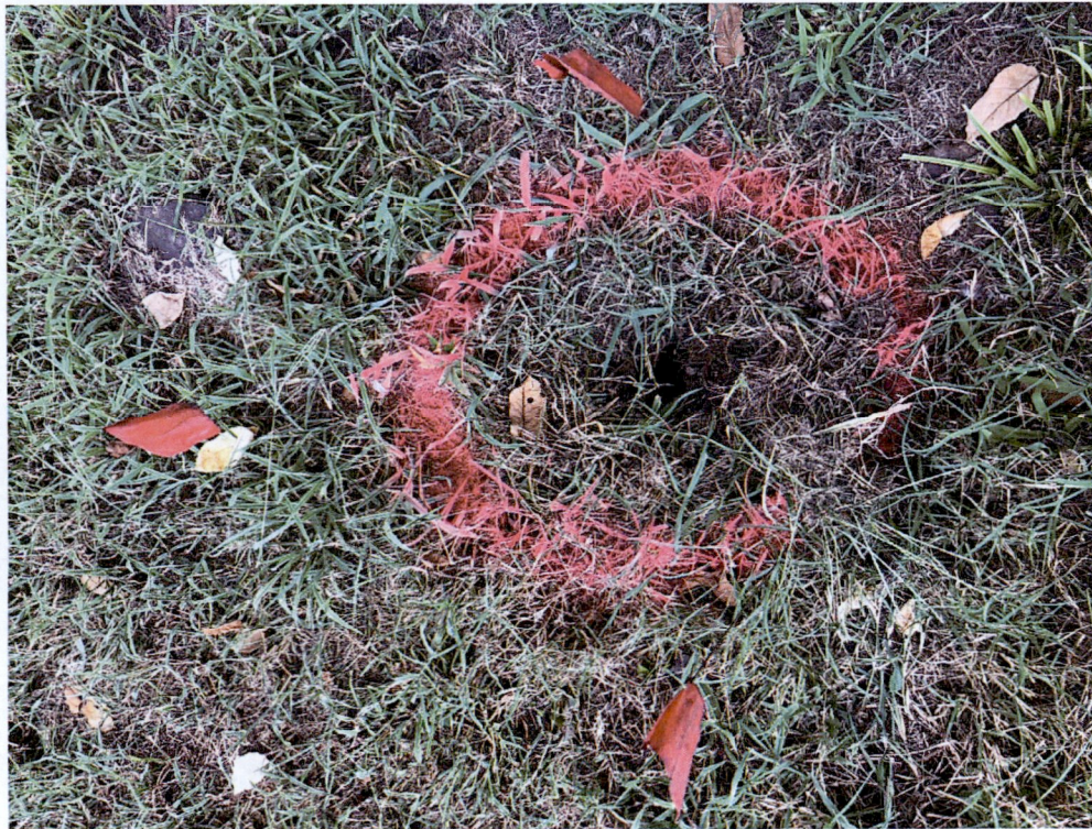
Private Service Line leaks that will require additional effort for repair.
