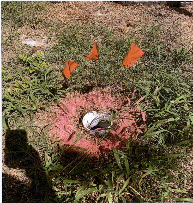
Typical Private Service Line Leaks that are easily corrected.
