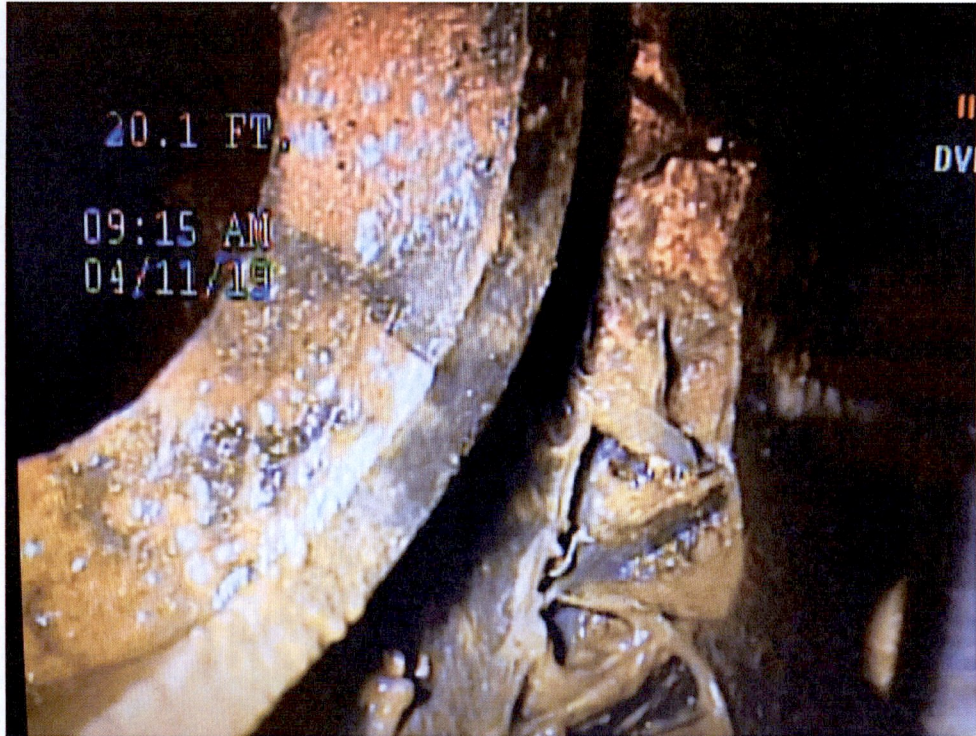
Service Line Tap into Truss pipe sewer Main, note the gap and failure to seal the joint
